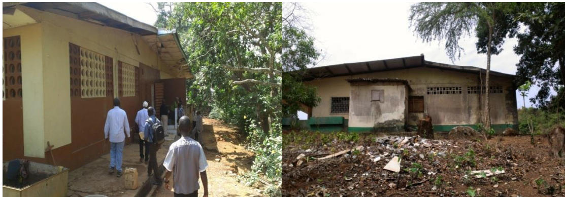
Figure 4. Villas in dilapidated state
