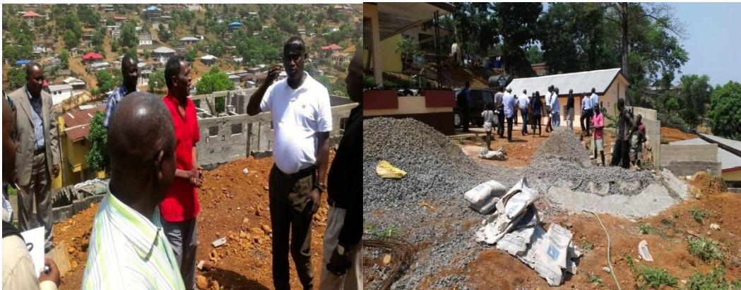
Figure 9. Committee Members cautioning tenants for undertaking massive construction works without the approval of the Corporation
