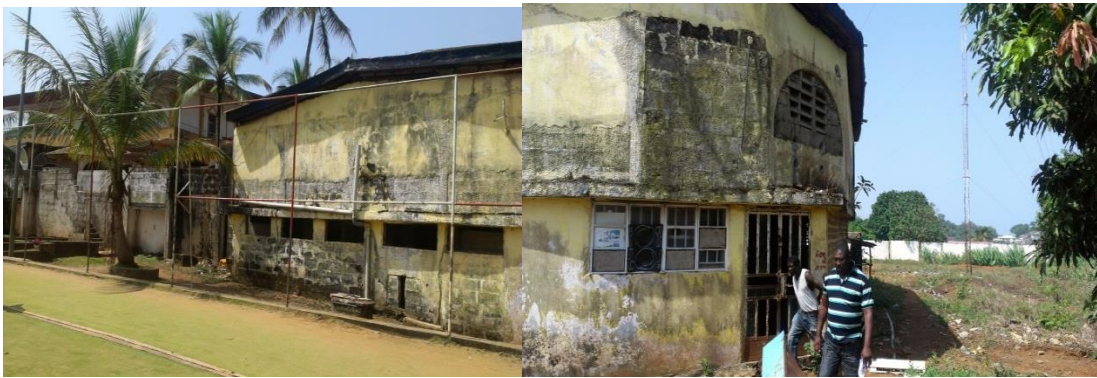
Figure 2. Back View of Old School Building in dilapidated State
